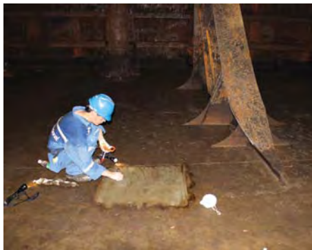
No.4 (S) - Lower: Excellent general condition of tanktop. Removal of residual oil layer from surface of coating.
