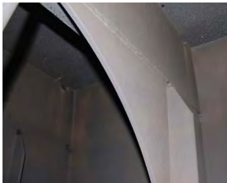
No.5 (S) - Upper: No breakdown on edges and weld seams on deckhead.
