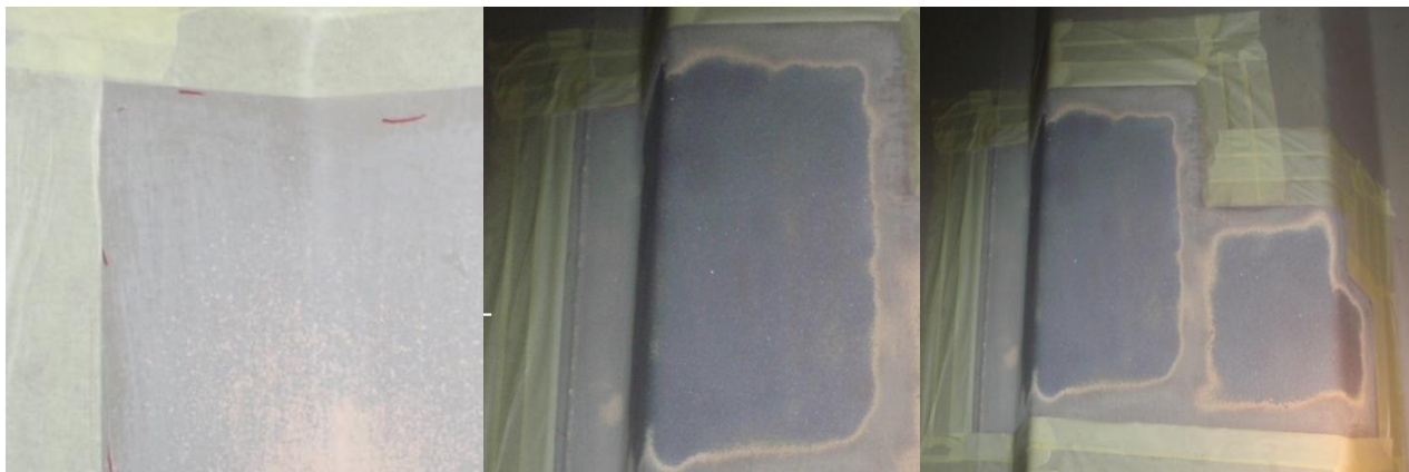
Examples of squared off areas, spot blasting and feathering back of intact coating
