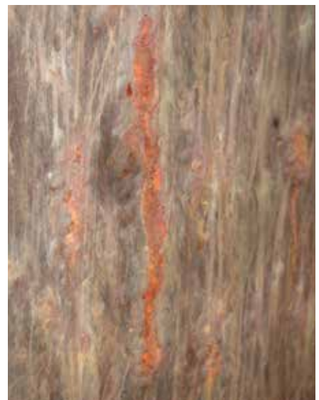
Images showing typical Cargo Hold Coating damage and subsequent corrosion caused by settlement
