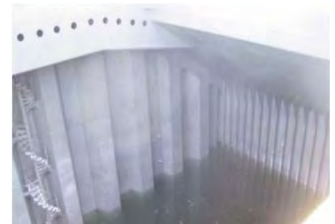
Ballast holds need excellent corrosion protection
