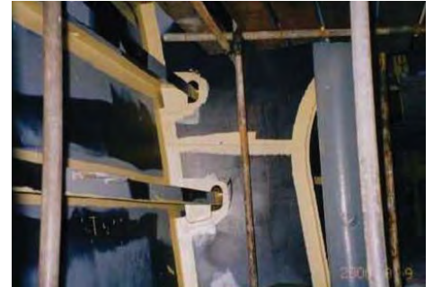
Touch up of Interbond®808 applied to bare steel plus one stripe coat to edges
