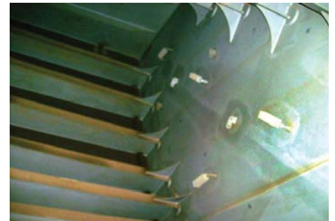
Excellent overall performance in water ballast tanks of a 159,000 DWT crude oil tanker after 5 years in service.
